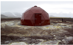
Wellhead in Krafla
